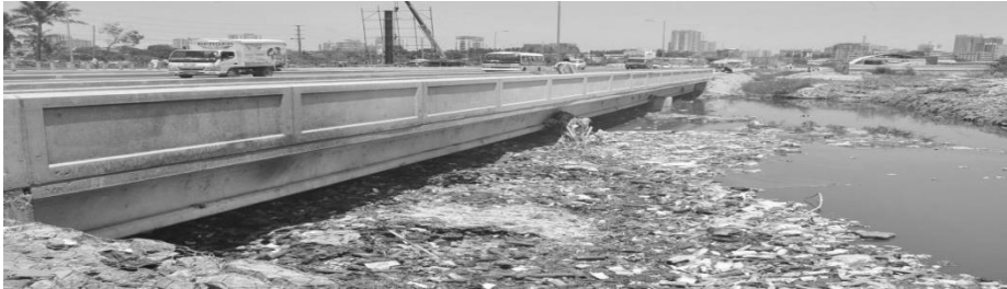
Figure 4.A Drainage System Filled with Solid Waste
